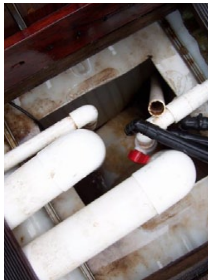
Pipework is hidden discretely under the decking and out of sight.
